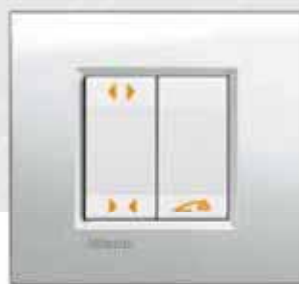
BLIND OPENING REGULATION AND BED HEAD AND BEDSIDE CABINET LIGHT LEVEL ADJUSTMENT PUSHBUTTONS
