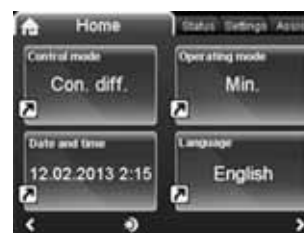
Fig. 1 Example of main display on a TPE Series 2000 with advanced control panel
