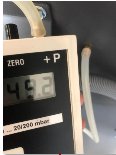
Pressure gauge connected to the measuring socket
