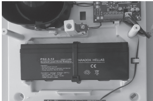
Figure 4. 2.7Ah battery installation
